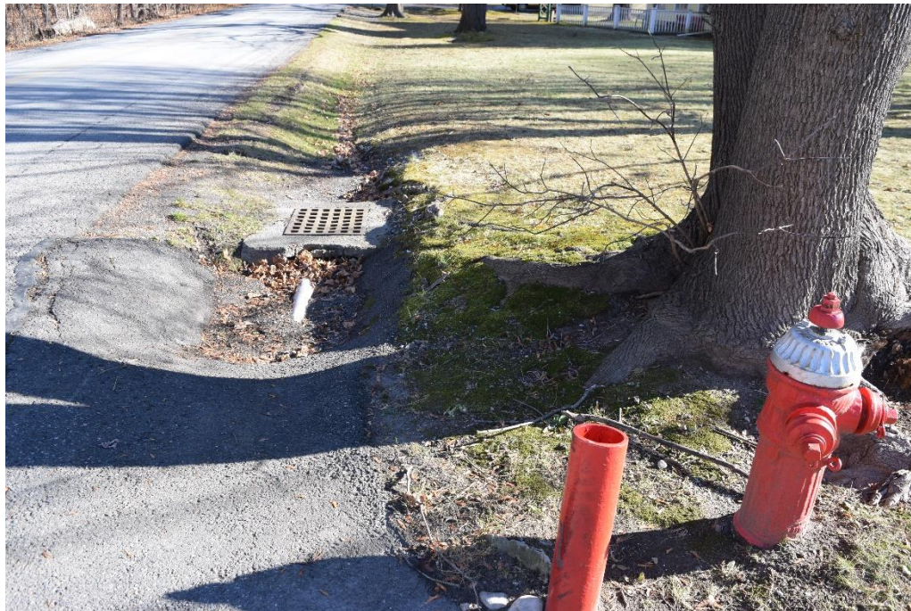
Photo 10. Close-up of the drainage grate and fire hydrant at the Hawks Avenue and Bank Street corner. View looking east-northeast.
